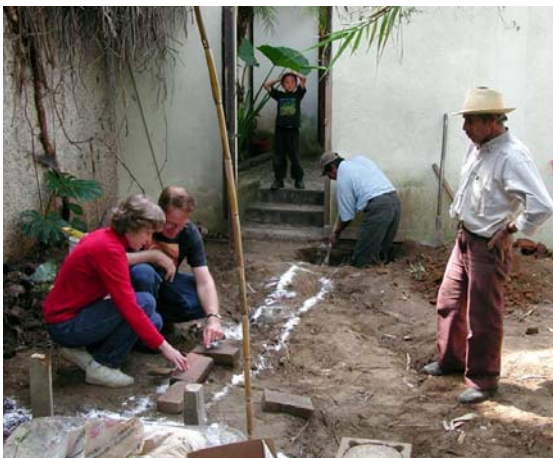
Mary and Paul McKay lay out bathroom with master builder, Moisés Hernández
